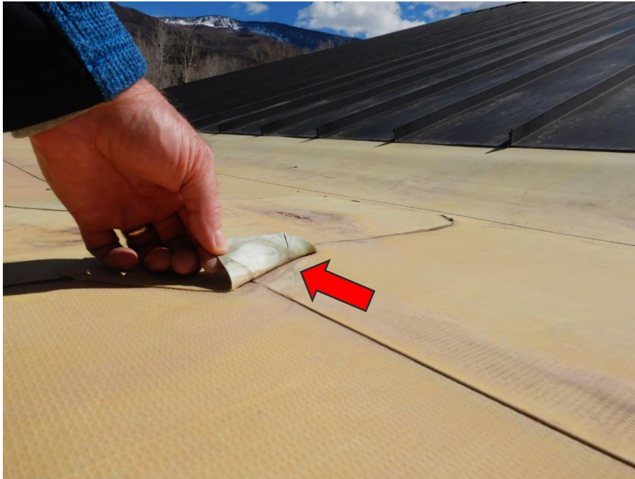
Figure 8. Debonded T-patch at TPO lap seam Roof F.
