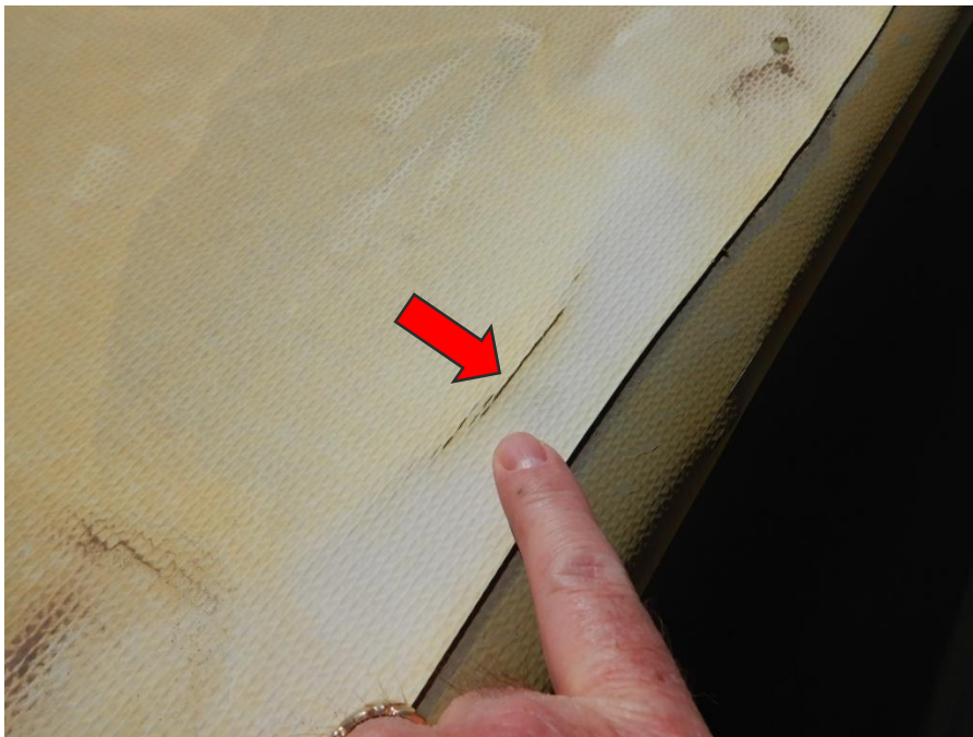
Figure 5. TPO membrane fracture at roof step down
