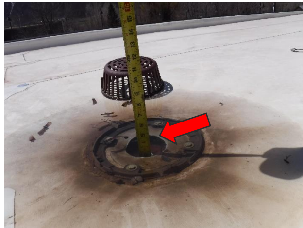
Figure 33. Approximately 4 inches of water.
