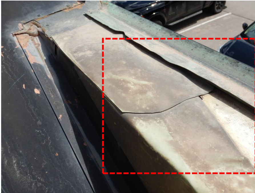
Figure 12. Stained pressure sensitive tape on south side of roof area F.
