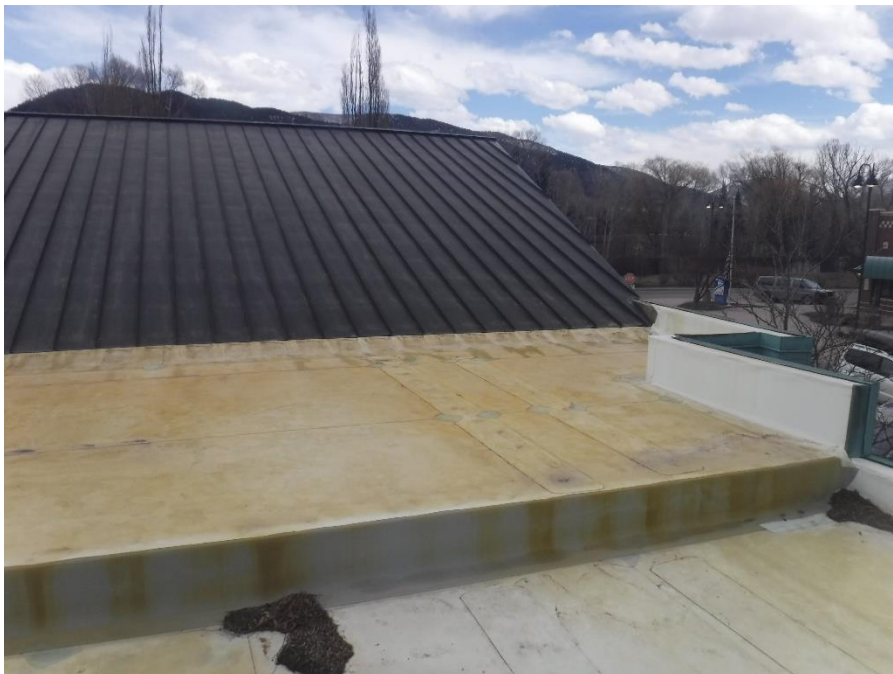
Figure 21. TPO significantly stained below copper roof.
