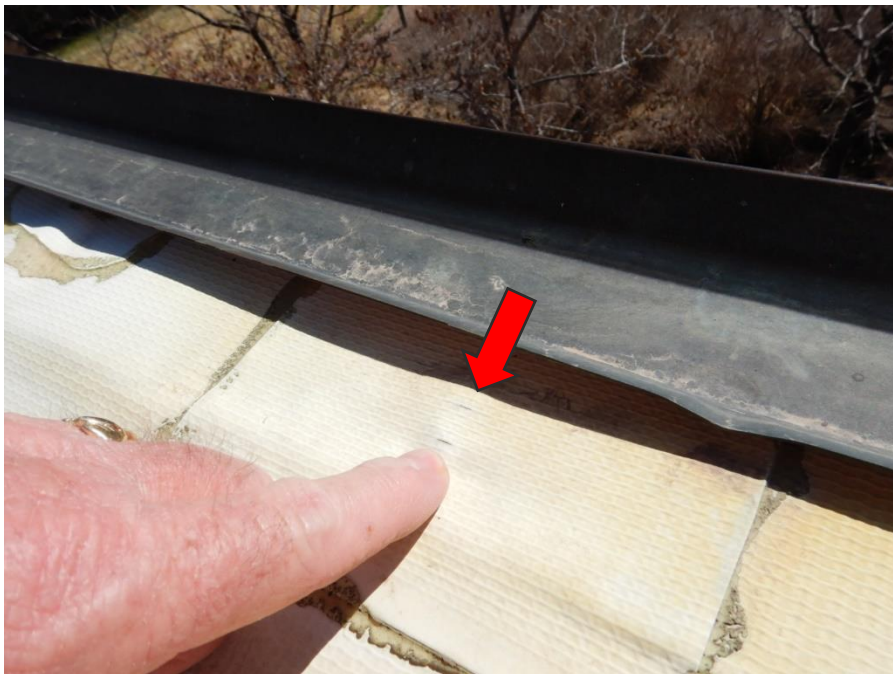
Figure 7. TPO membrane deterioration at parapet wall.
