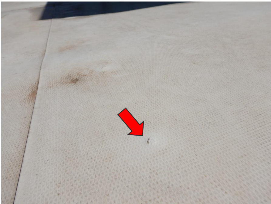
Figure 17. Fastener head under TPO membrane with damaged membrane surface above.
