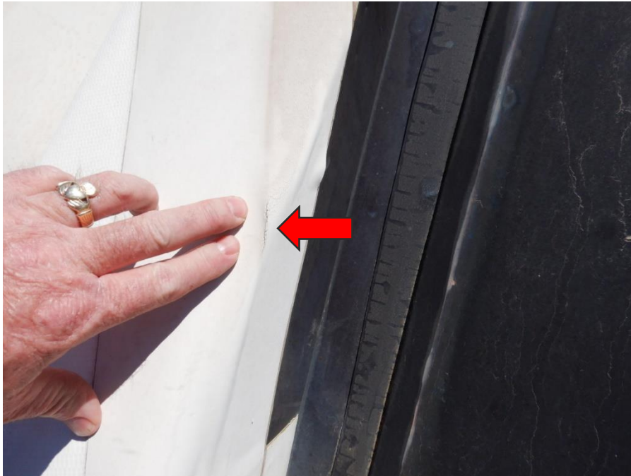
Figure 6. Deteriorated pressure sensitive tape over metal flashing.
