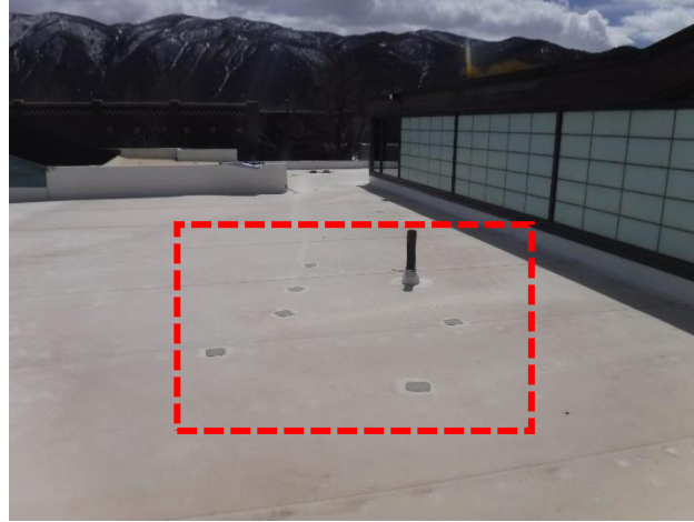
Figure 23. Numerous repair patches.
