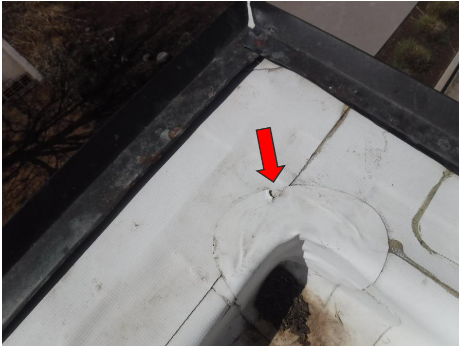
Figure 18. Inside corner T-patch is torn.
