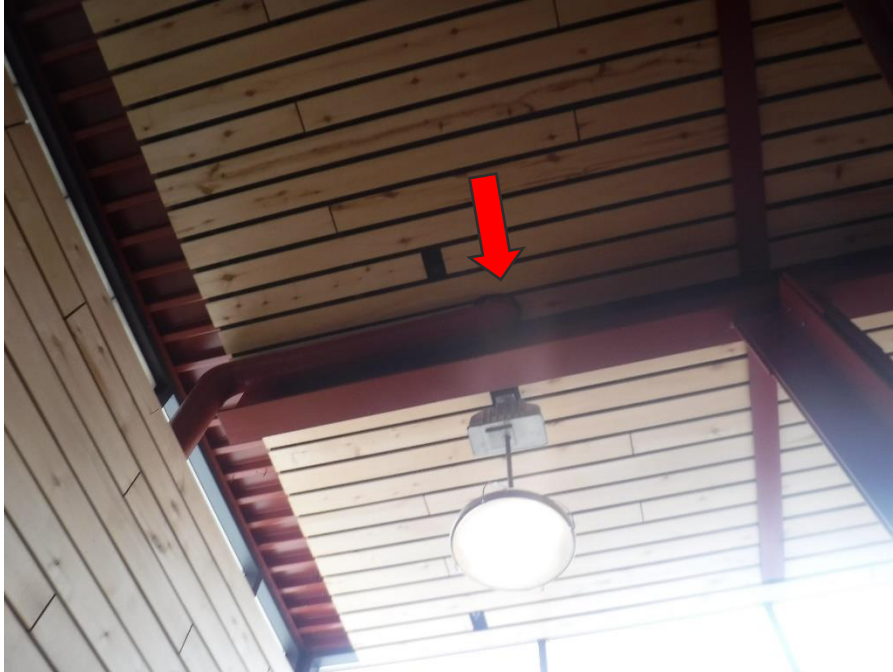
Figure 31. Roof drain penetration located adjacent to column where there were reported leaks.
