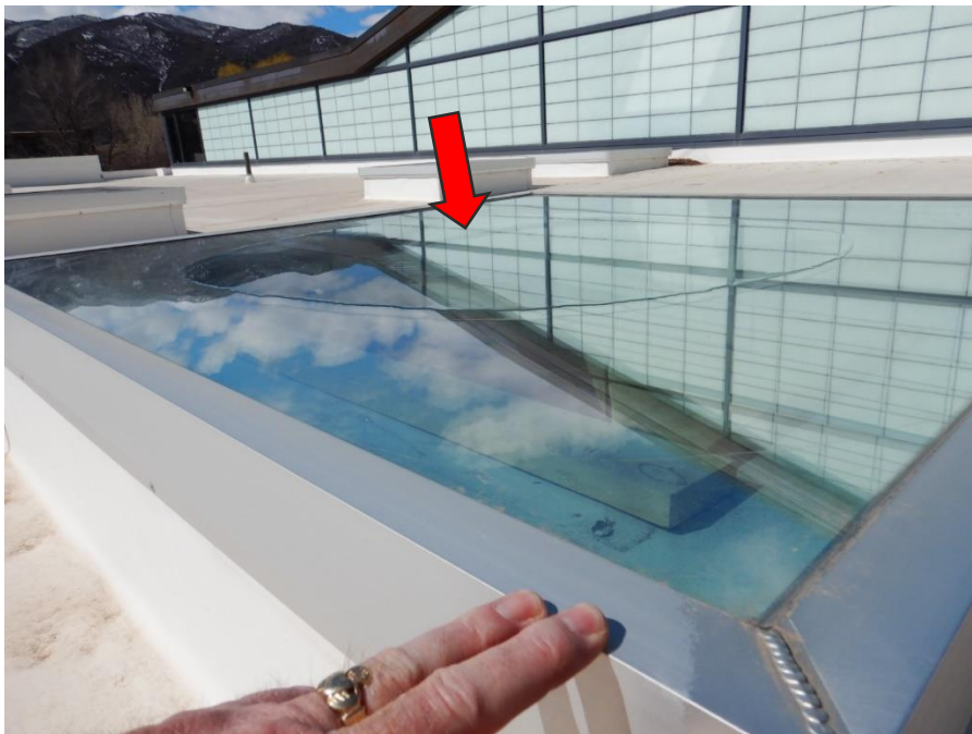
Figure 19. Ponding water on the skylight.
