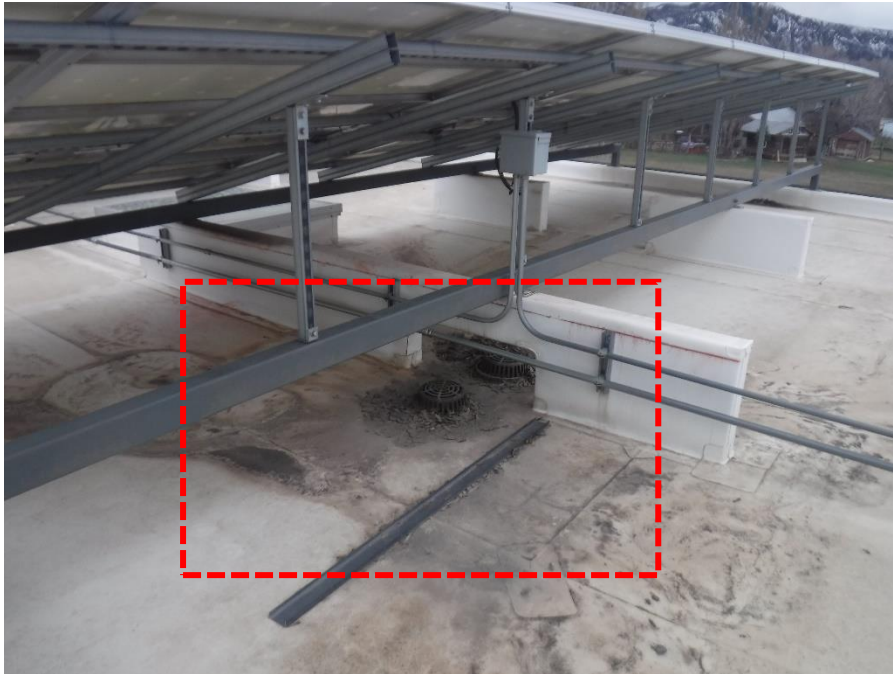
Figure 20. Staining from water and debris accumulation.
