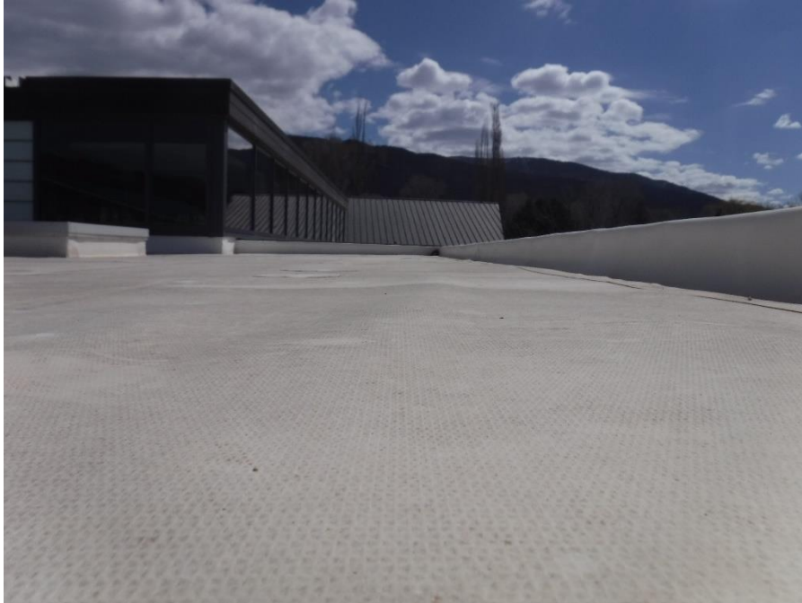
Figure 4. The reinforcing scrim is visible through the surface of the TPO membrane.
