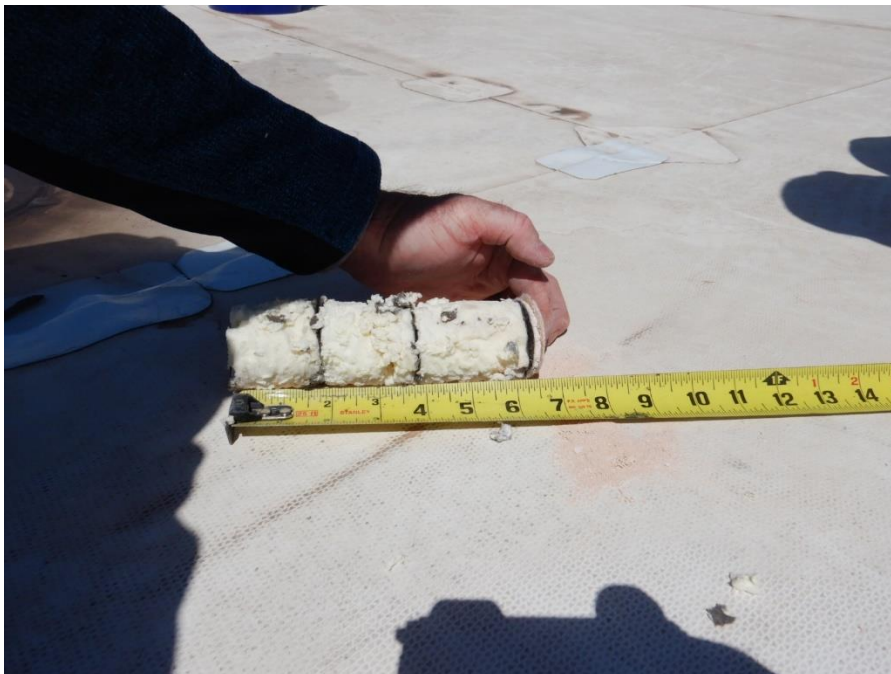
Figure 28. Core section of the roofing system. Starting from left, three layers polyiso insulation, and cover board.
