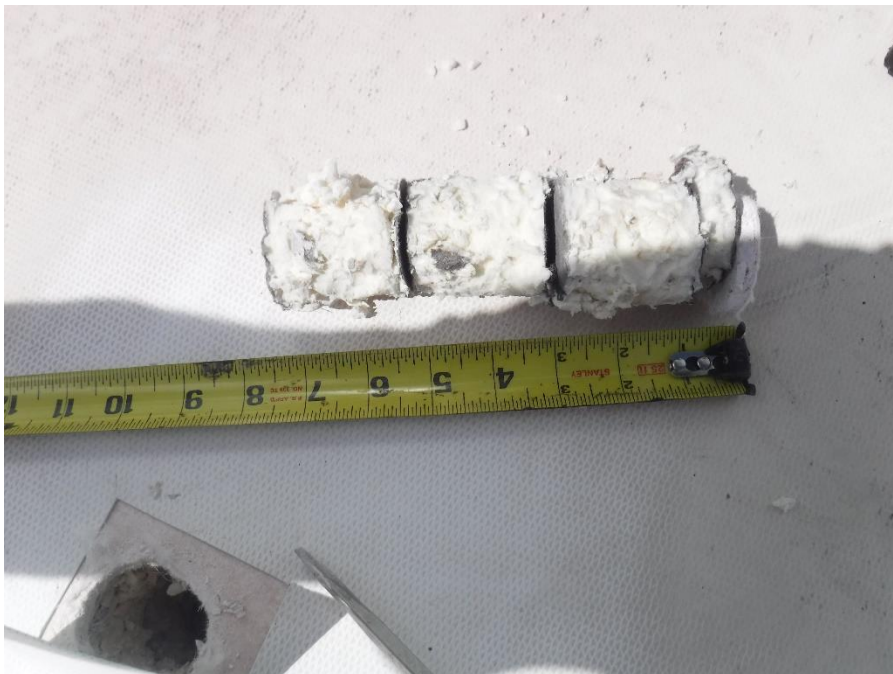
Figure 26. Core section of the roofing system. Starting from left, three layers polyiso insulation, tapered insulation and cover board.
